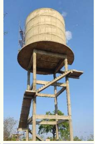
Overhead Water Tank that was built recently in the village under Narmada-Parvati River Linking Project
